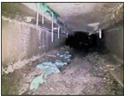
SEE VIDEO FOOTAGE FROM INSIDE THE BROKEN MORRISON BRIDGE DECK AT PORTLANDMERCURY.COM
